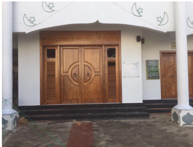
Damaged mosque in Kohilawatta,Wellampitiya
